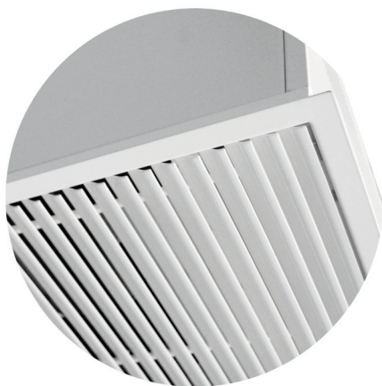
Detail of exposed inlet grille
